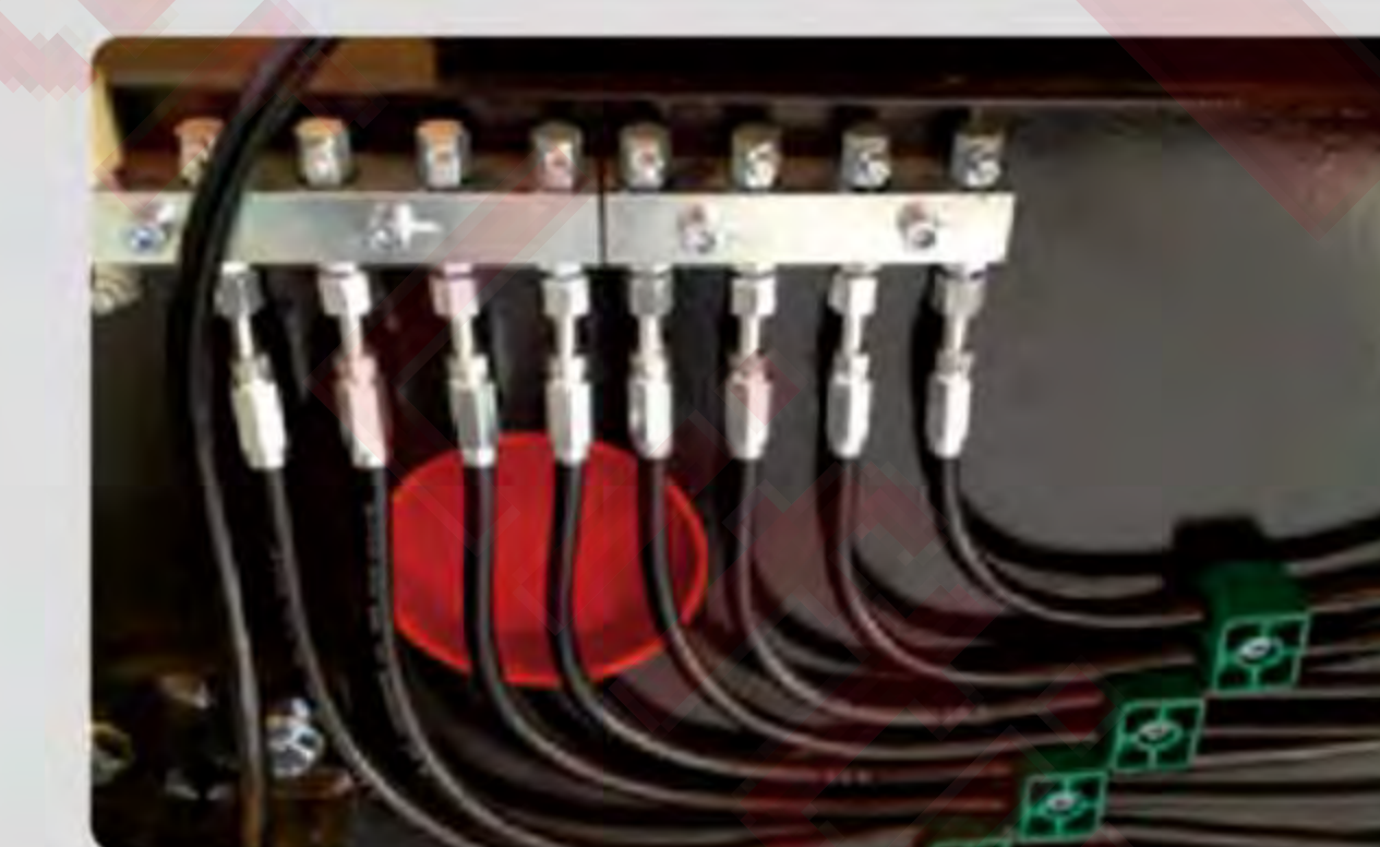
Centralized Lubrication System
